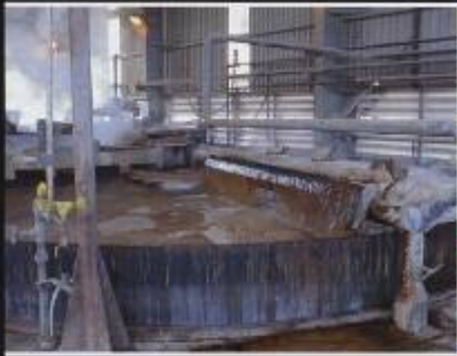
Filter in operation for over 20 years
